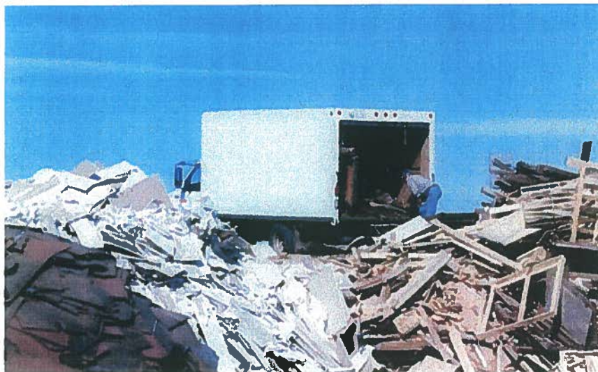
C&D waste accounts for a quarter of the waste generated in Alberta. Four to seven tonnes alone (six 12-yard bins) is produced from an average house construction.
